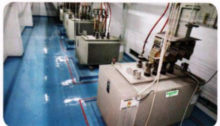
Thamrin City, Shopping Centre and Apartement, Jakarta - Indonesia
